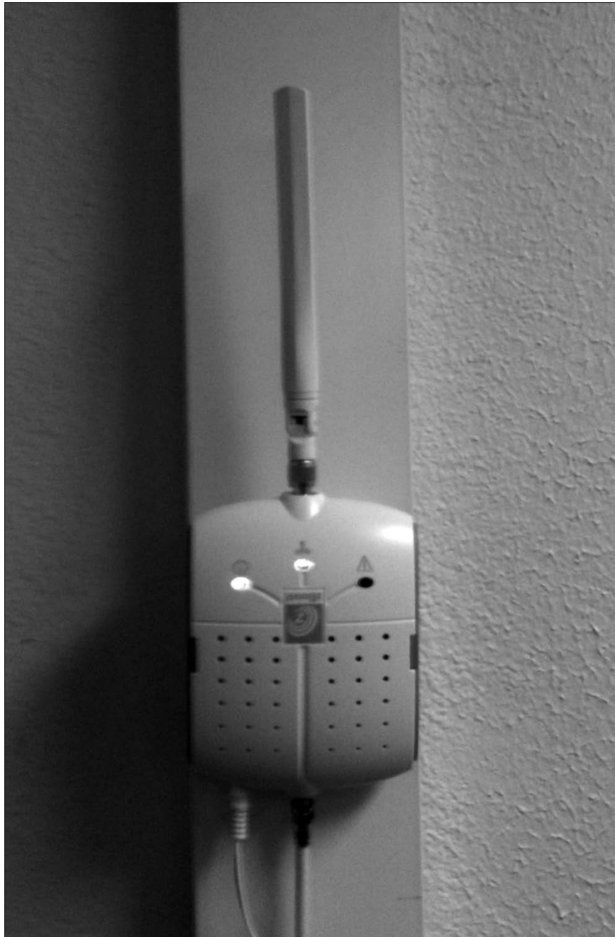
Figure 12-4: This device boosts signals on the two most common cellular frequencies to improve reception in an office located between two large buildings.
